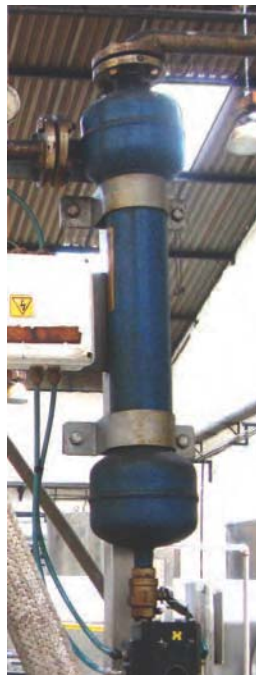
ILB removes solids in a food processing plant.
