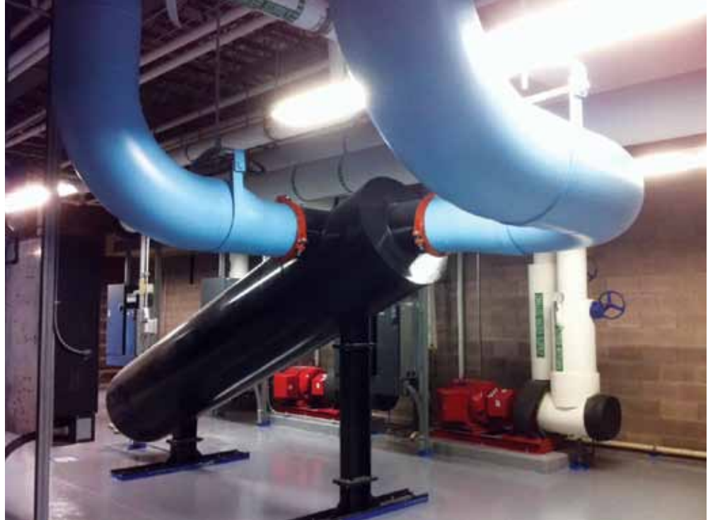
LAKOS HTH 3500 used to keep wind-blown sand from damaging heat exchangers and other equipment in manufacturing plant in New Mexico.
