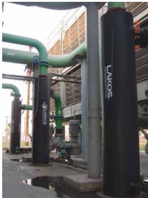
Series of LAKOS HTH 1950 separators used to keep sand out of customer cooling tower installation in Mexico.
