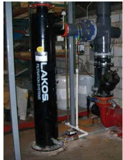
LAKOS HTH 0500 used to keep water tower condenser free of solids in chilled water system.
