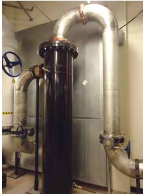
HTX installed at Peppermill Casino in Reno, Nevada, keeps their geothermal heat exchanger clean and free of dirt. The Peppermill has won numerous awards for its facility, including Green Company of the Year
