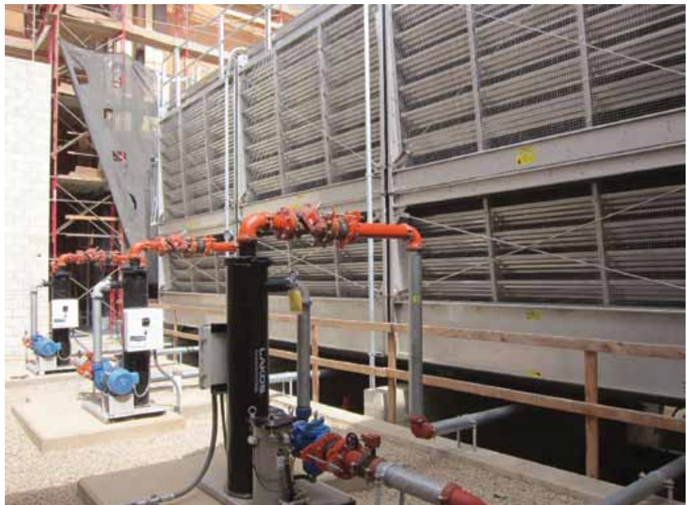
LAKOS HTX Separators on packaged TCX systems keep this cooling tower clean at a Resort and Spa in Hawaii
