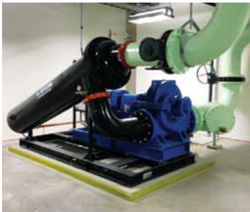
Side Stream Filtration, Parkland Hospital, Texas USA
