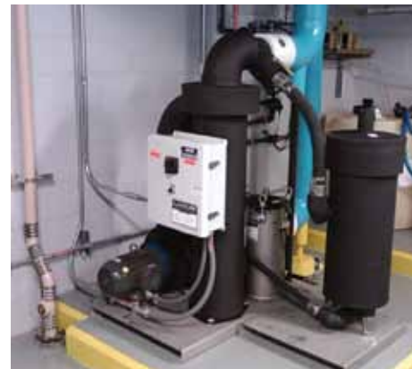
Closed loop Filtration, Data Center, Virginia USA
